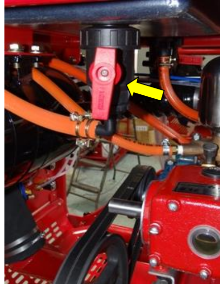
Before opening the filter shut the formulation line ball valve (shown here in open position).
