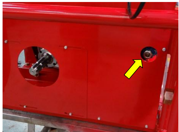
Blower oil level indicator (gear drive side).
